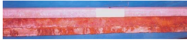
Fig 1: Corrosion damaged beam
