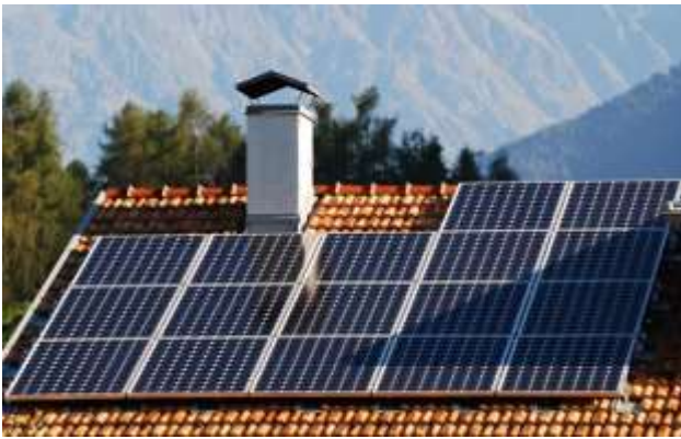
Fig 2: Partial Shading on Photovoltaic Panels
