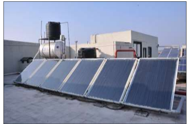
Fig 9: Solar water heater
