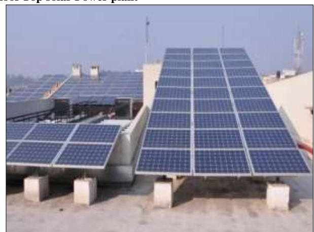
Fig 7: Solar Roof top power plant
