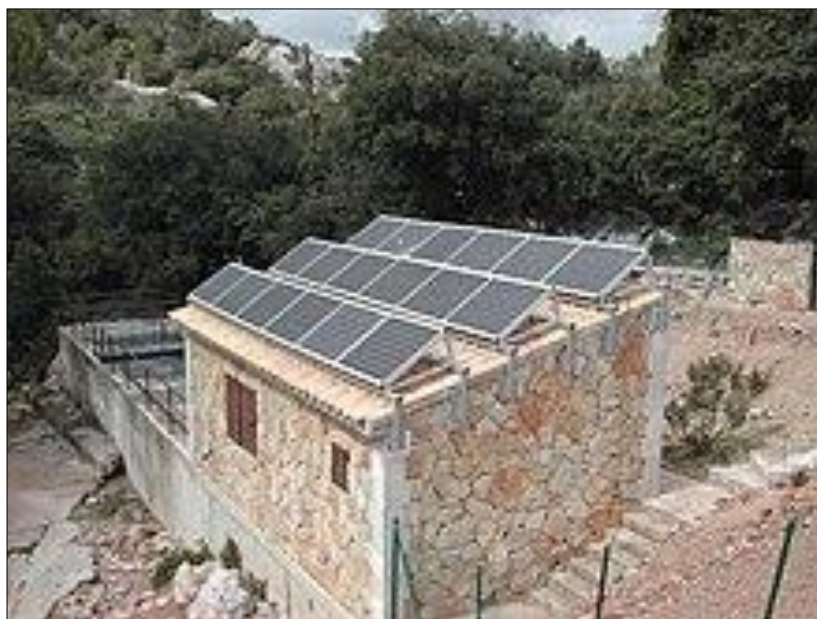
Fig 5: A sewage treatment plant that uses solar energy, located at Santuaride Lluç monastery, Majorca.
